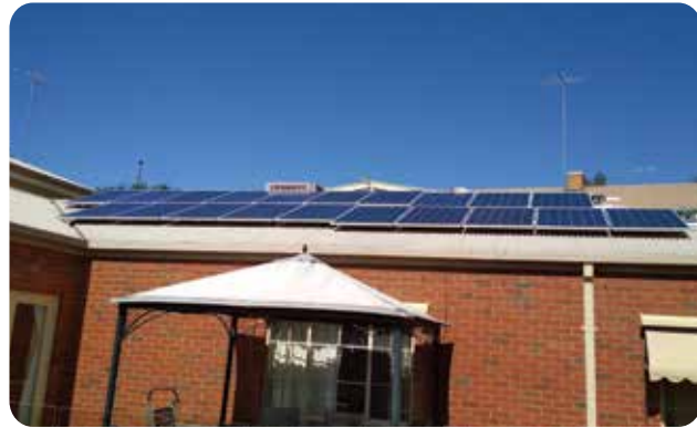
Location: Melbourne, Australia Capacity: 6KW Model: MG6KTL
