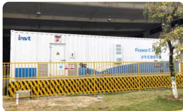
Location: Guangdong,China Capacity: 500kW/1.8MWh Model: BD500KTR-T
